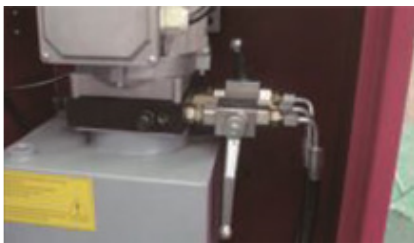
Main hose joint in the middle, and leveling hose joint on the each side
